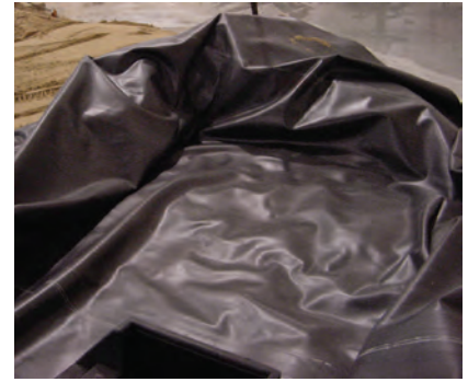
The liner covers the stream bed and goes thru the area where the spillway will set.
