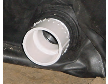
Bulkhead is thru liner, washer and nut are tightened and PVC adapter is installed.
